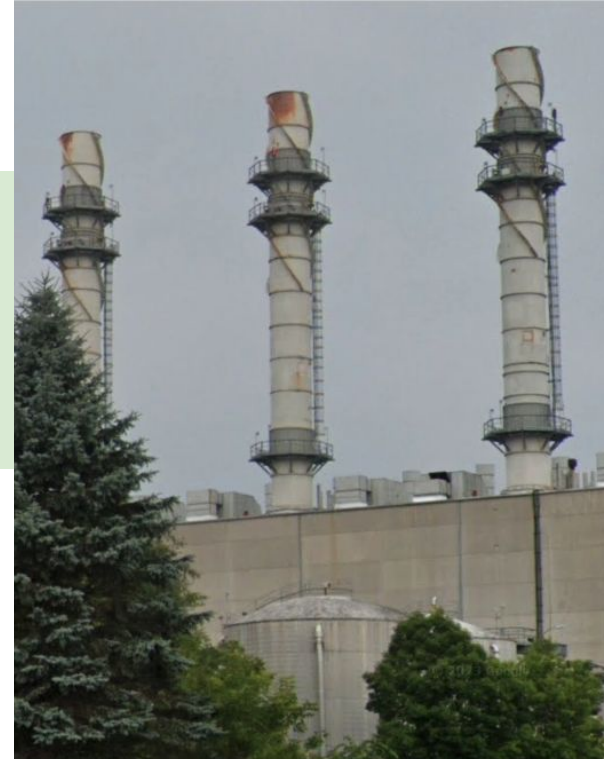
Declining conditions at Berkshire Co's last large fossil fuel peaker power plant.
